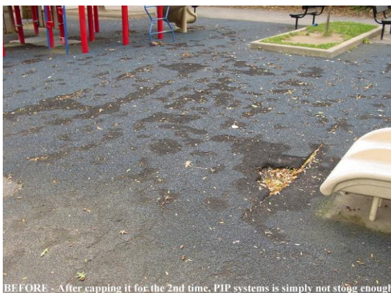
BEFORE - After capping it for the 2nd time, PIP systems is simply not strong enough
